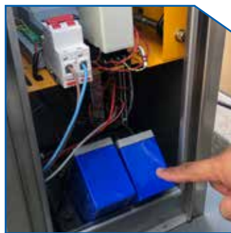
Backup battery keeps barrier running while power off
